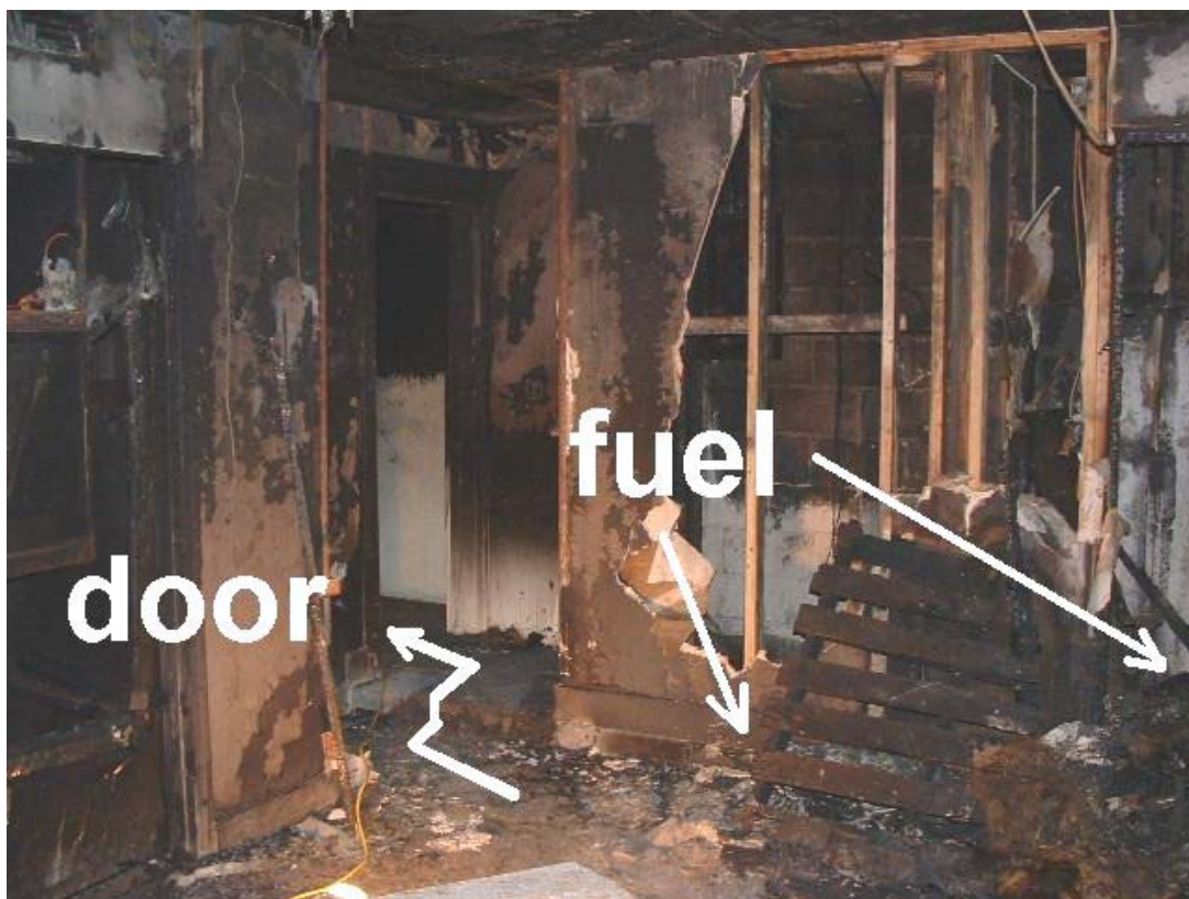
Figure 1: Photo looking SW showing fuel proximity to only doorway
