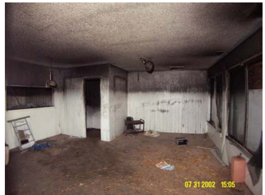
Figure 7 - living room near front entry looking towards doorway used to enter/exit the first of two small rooms before the fire room (see floor plan)
